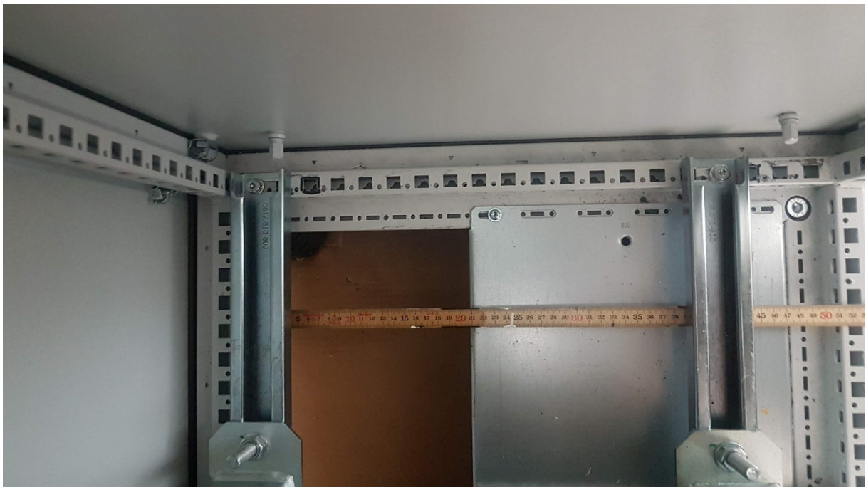
Figure 7 opening at the bottom of the cabinet (top view from inside). About 1/3 remain open.
